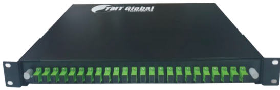
24 PORT SLIDING TYPE FIBER PATCH PANEL WITH SC/APC SIMPLEX ADAPTER
